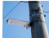
防犯灯・街路灯 LED 化
